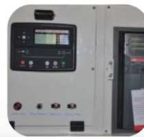
Control Panel & MCB
